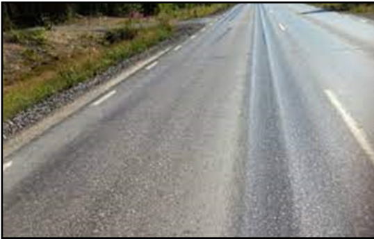
A badly rutted carriageway
